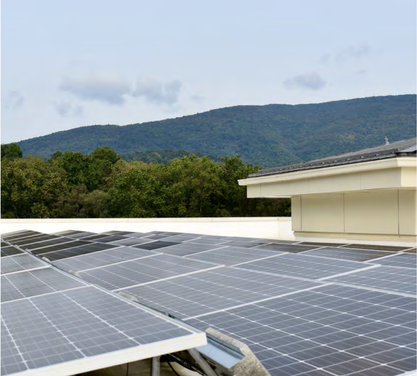
(Above) Solar panels on the Crozet Library.
